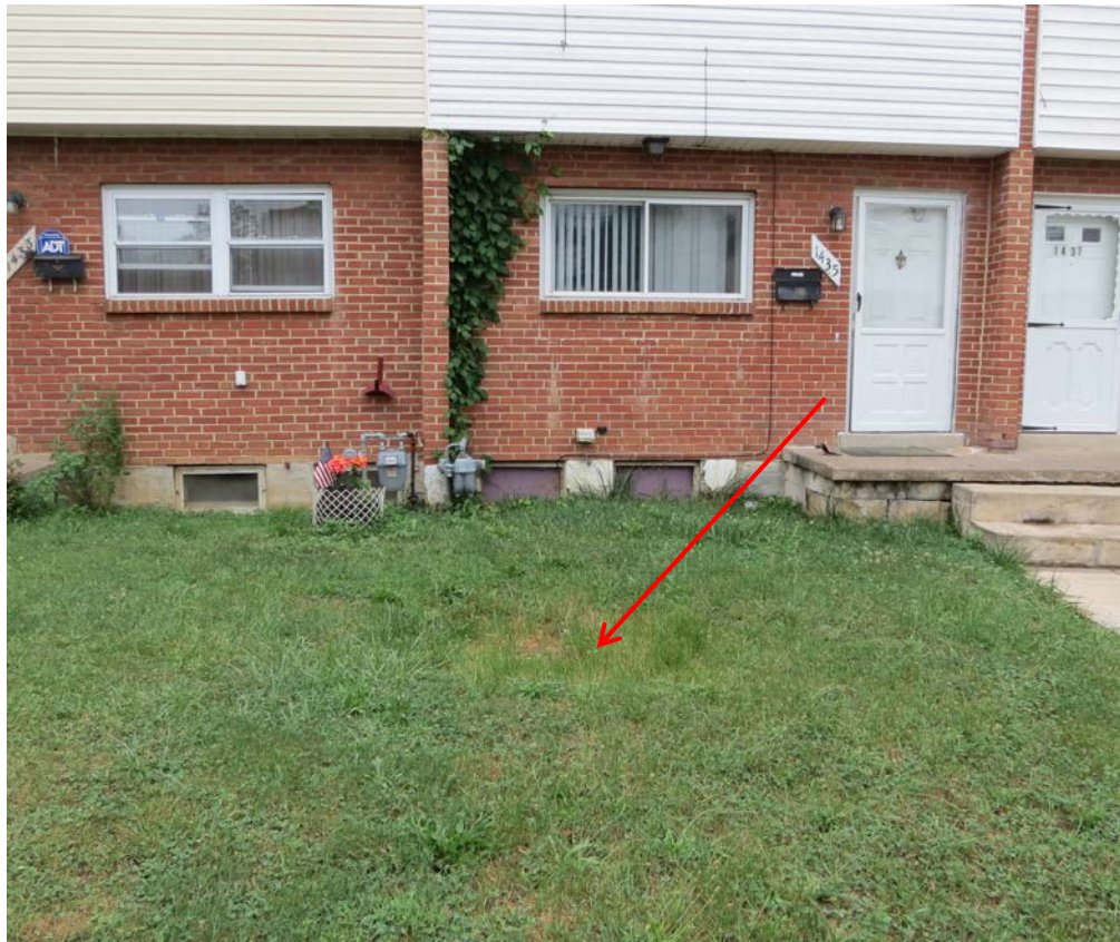
S. 14 th Street – Photo 6 Surface Depression in Front of House No. 1435
