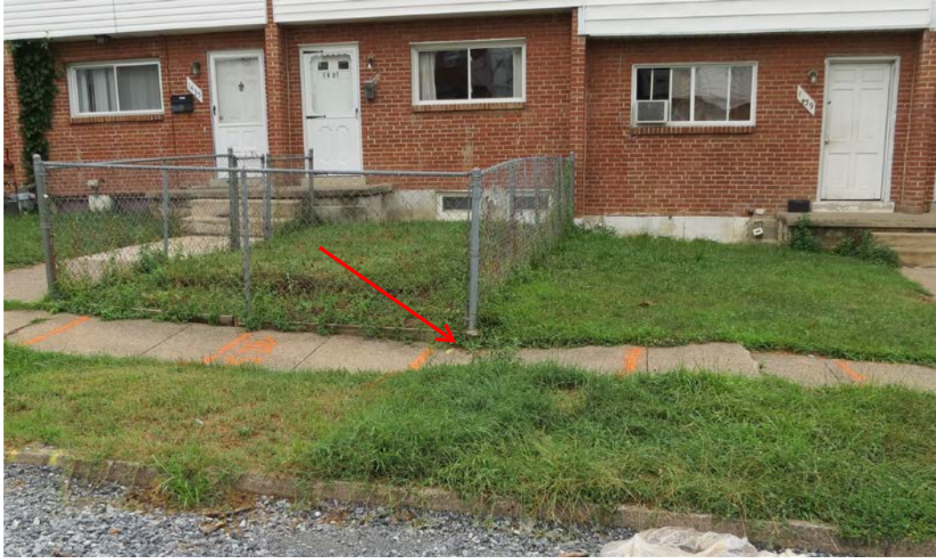
S.14 th Street – Photo 3 Sidewalk Sag Between House Nos. 1437 and 1439
