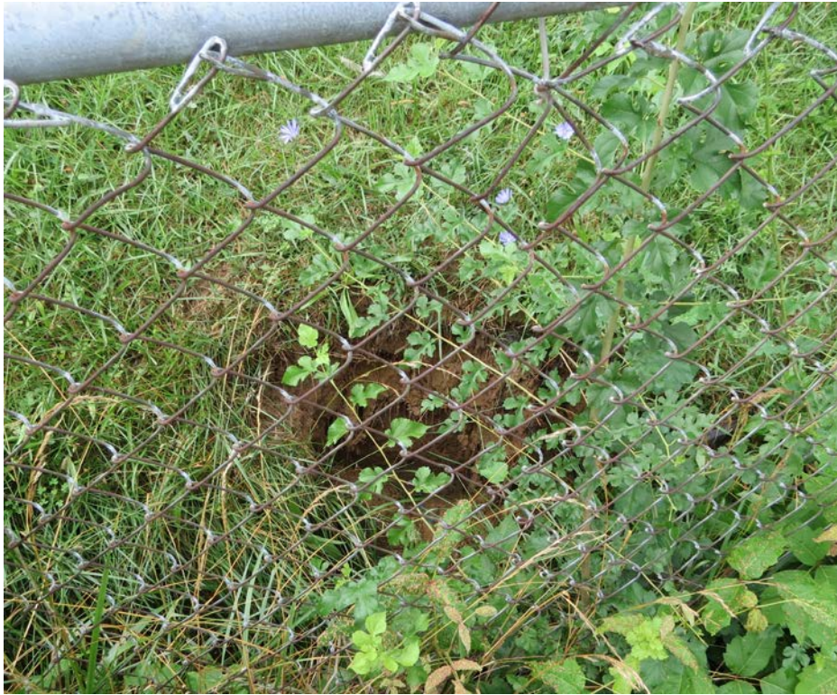
S. 14 th Street – Photo 8 Sinkhole in Front of House No. 1426
