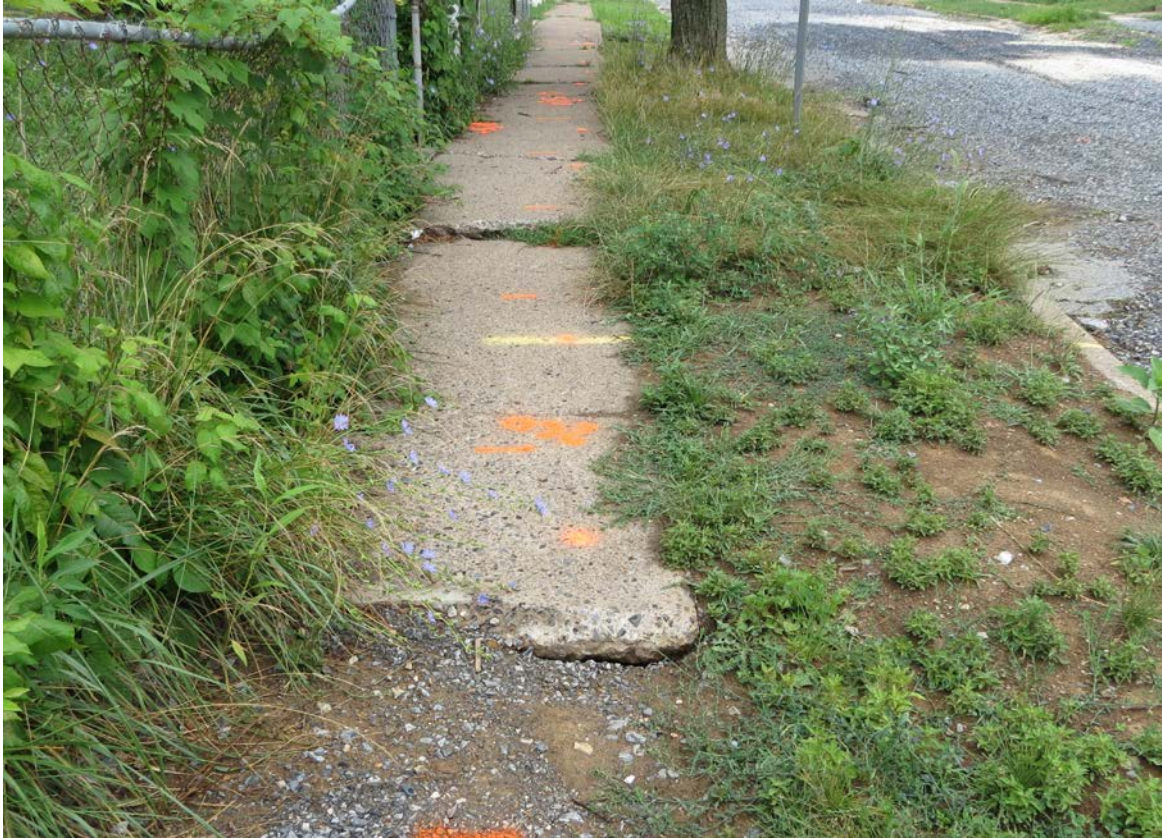
S. 14 th Street – Photo 9 Depressed Sidewalk in Front of House No. 1426
