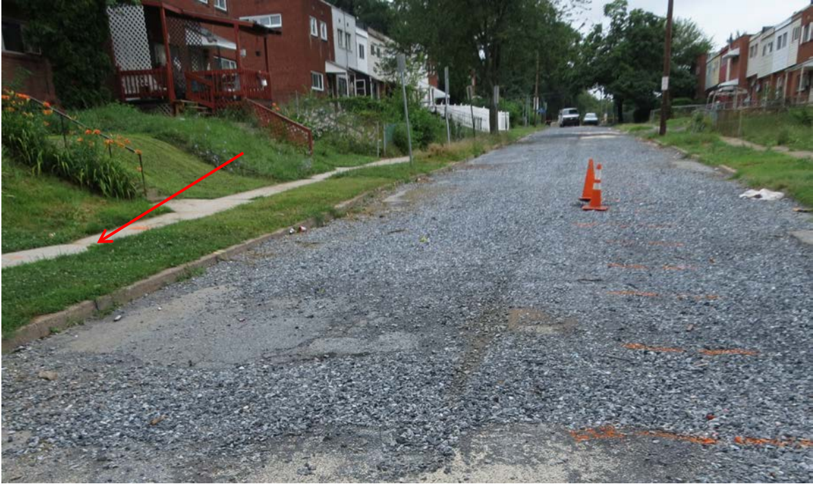
S. 14 th Street – Photo 1 Sidewalk Sag on Left in Front of House No. 1440
