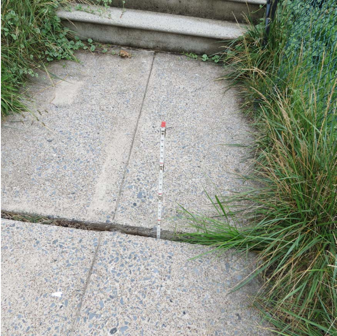
S. 14 th Street – Photo 13 Approximate 11" Void Depth Below Entrance Sidewalk at House No. 1423
