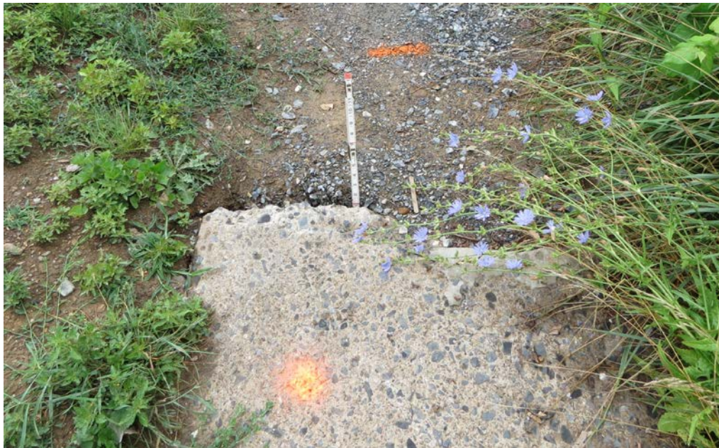
S. 14 th Street – Photo 10 Approximately 1'-1" Void Depth Below SW Slab in Front of House No. 1426
