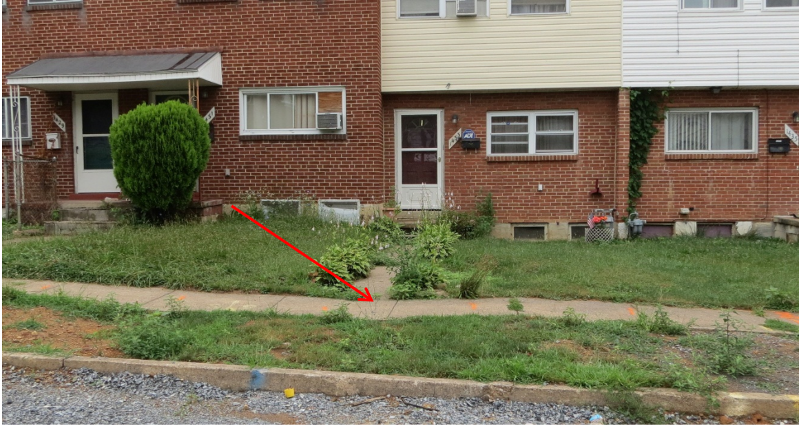
S. 14 th Street – Photo 5 Sidewalk Sag in Front of House No. 1433
