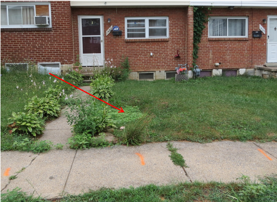
S. 14 th Street – Photo 4 Surface Depression in Front of House No. 1433
