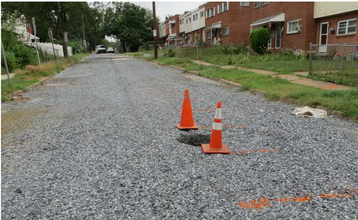
S. 14 th Street – 2 Sinkhole Opened During MASW Testing Between House Nos. 1436 and 1439
