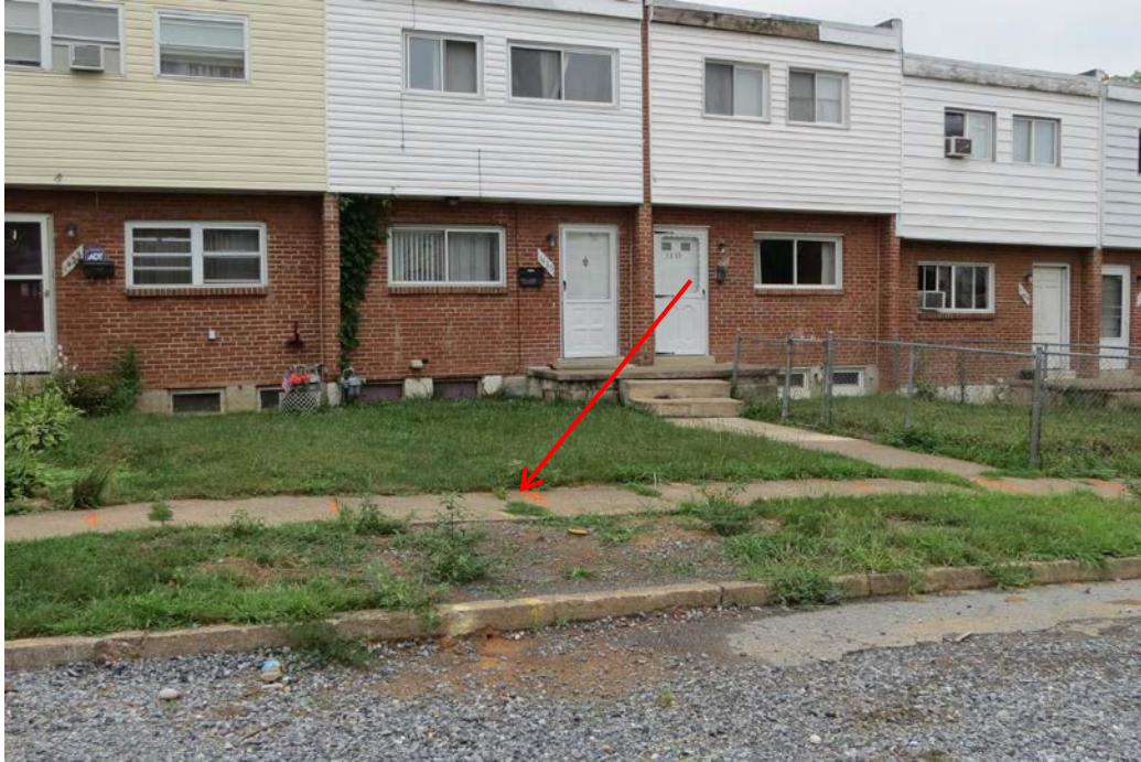
S. 14 th Street – Photo 7 Sidewalk Sag in Front of House No. 1435
