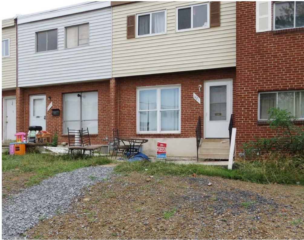
S. 14 th Street – Photo 12 House No. 1421, Location of 1985 Structural Foundation Repair with Evidence of Recent Subsidence
